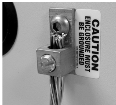
Figure 6. Ground terminal on bottom of the enclosure.
