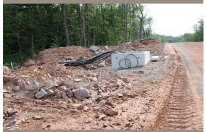
Pre-cast concrete vault for underground collector circuit isolation switch.
