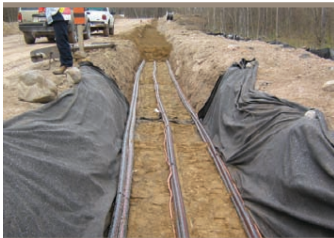
Prince 1 underground collector system.
