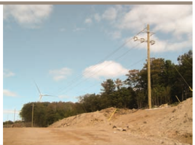
Prince 2 overhead collector system.
