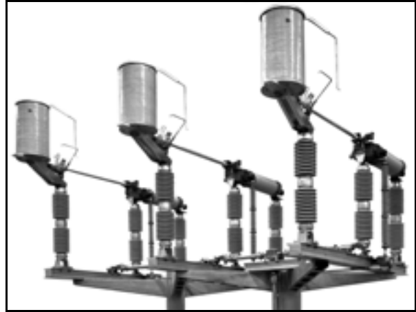
Figure 2. High-resistance pre-insertion inductors mounted on a 138-kV Mark V Circuit-Switcher.
