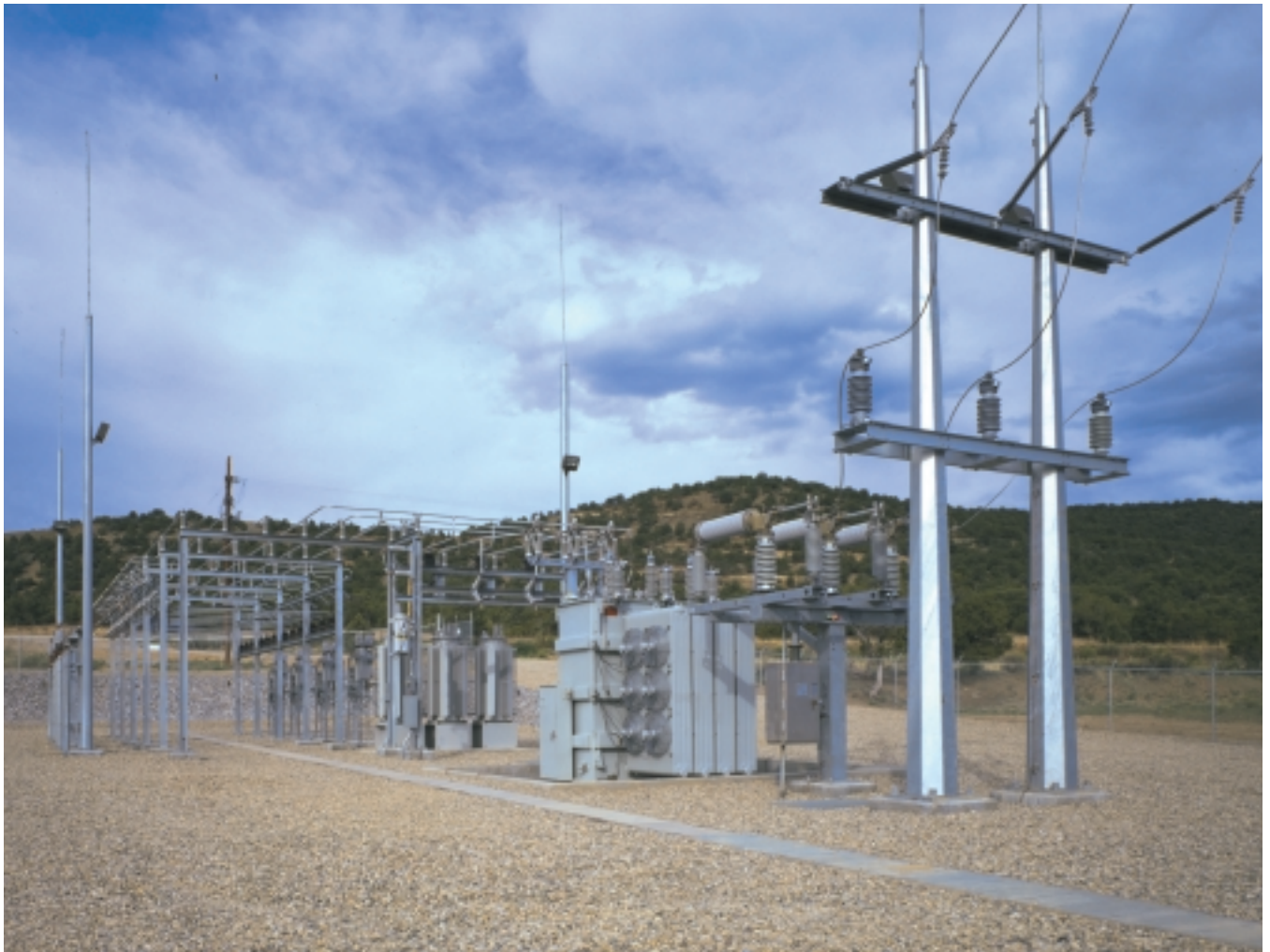
Figure 1. Distribution substation in southwestern United States featuring more than one hundred forty Cypoxy station post insulators for apparatus and bus-support applications.
