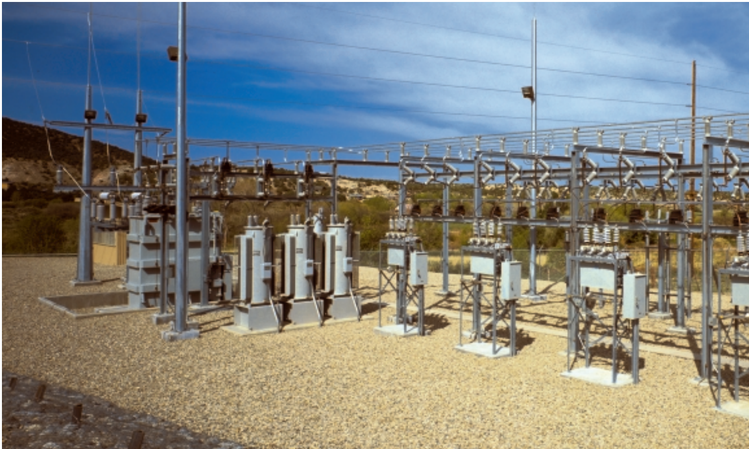
Figure 2. . . . another view of substation showing the extensive application of S&C's Cypoxy station post insulators.
