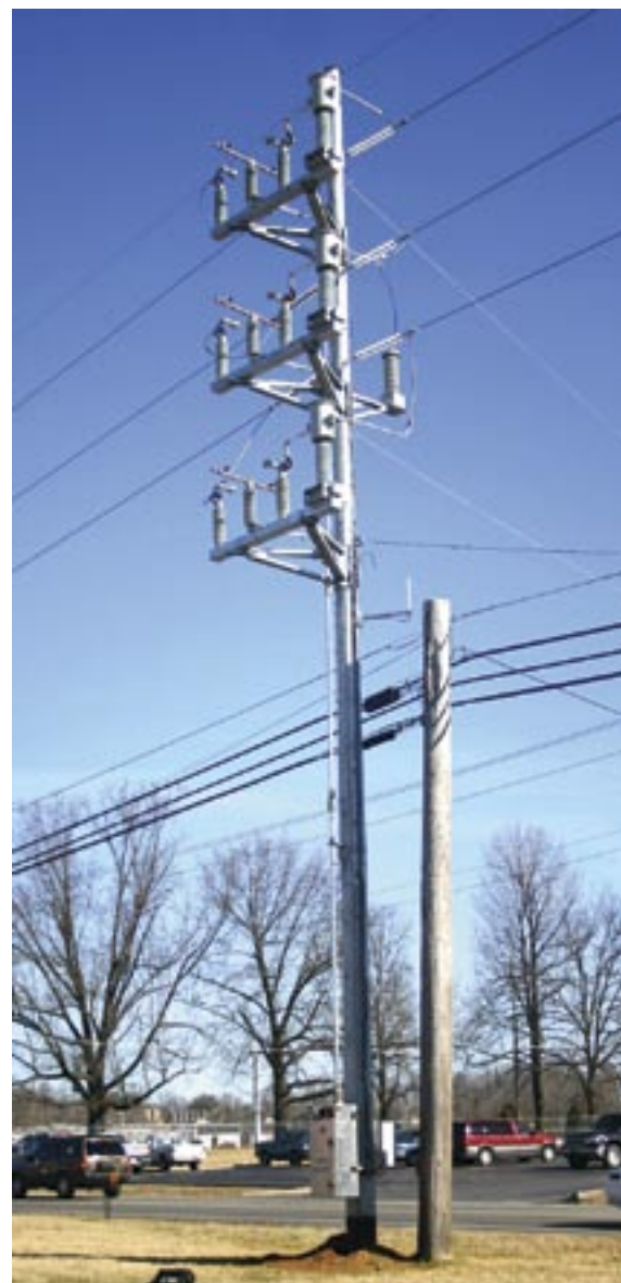
69-kV Double-Break Style Alduti-Rupter Switch in the Tiered Upright Mounting Configuration.
