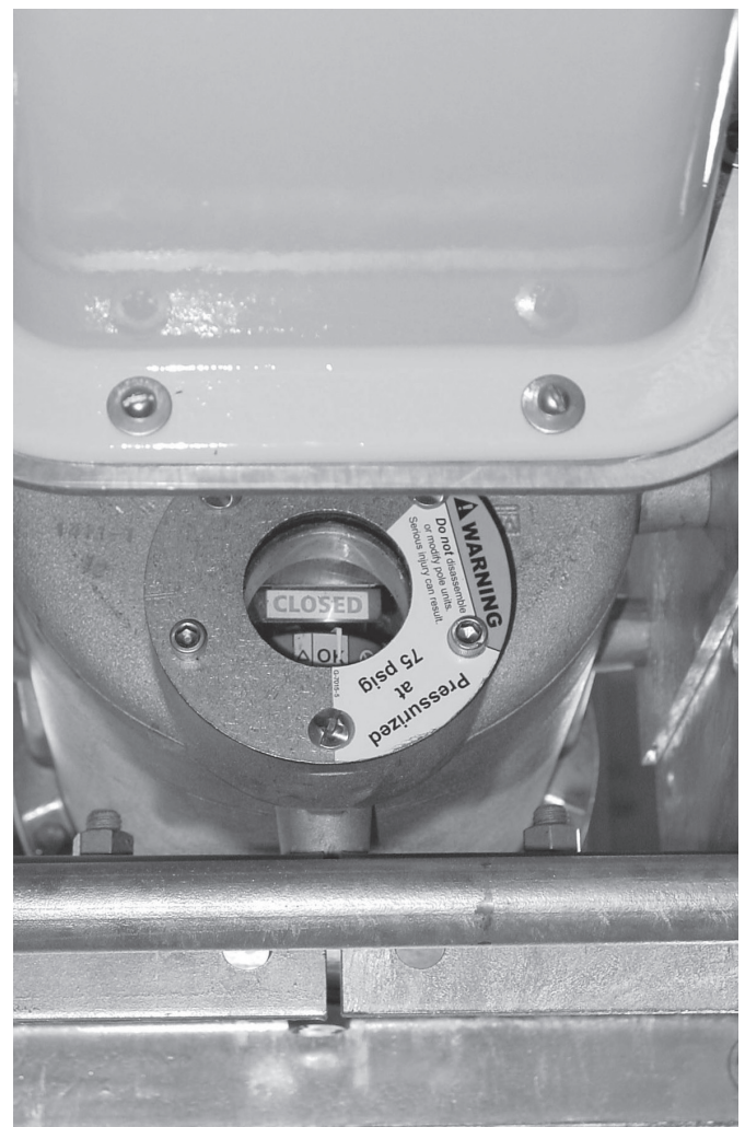
Figure 3. Indicators are fully visible beneath a pole-unit with motor operators installed.
