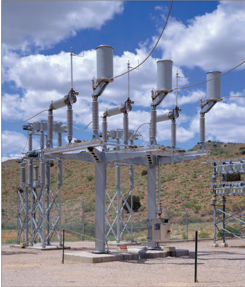
Pre-insertion inductors mounted on 138-kV Vertical-Break Style Mark V Circuit-Switcher.
