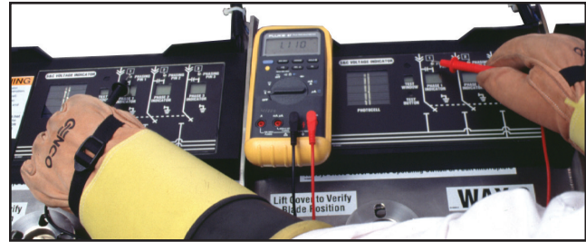
Figure 3. Measuring the phase-to-phase voltage—Phase 1 to Phase 1—using an optional potential indicator with a low-voltage phasing feature.)
