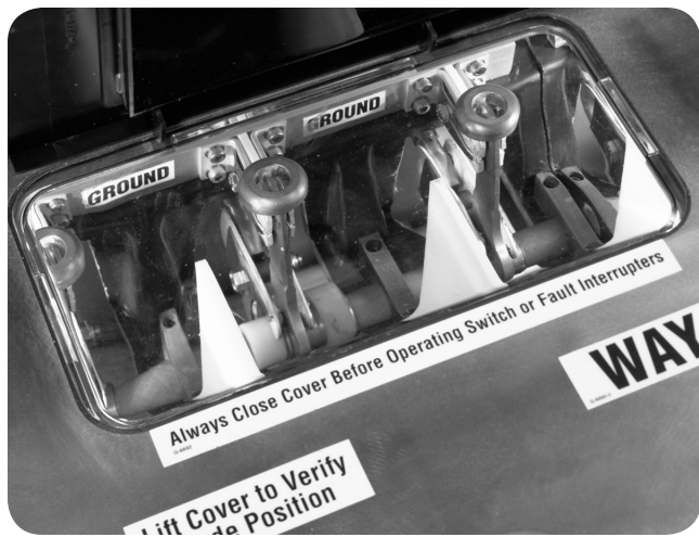
Fault interrupter shown in ground position... cables are now solidly—and internally—grounded.
