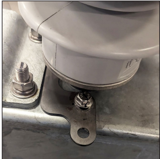
Figure 7. Lower bracket and bolt installed, not tightened.
