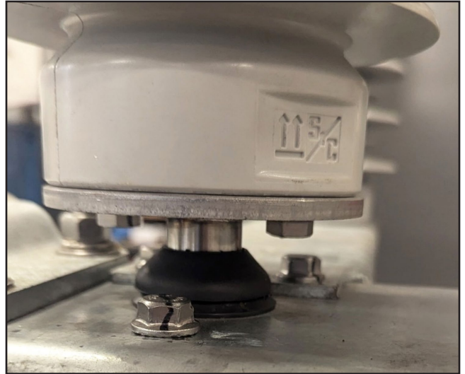
Figure 4. Bottom of the post insulator in the Closed position.
