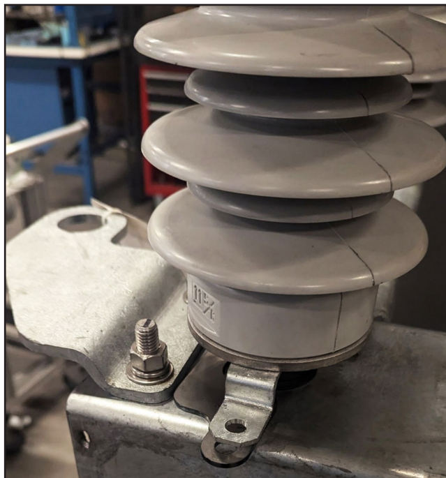
Figure 11. Aligning the lower bracket hole with the upper bracket.
