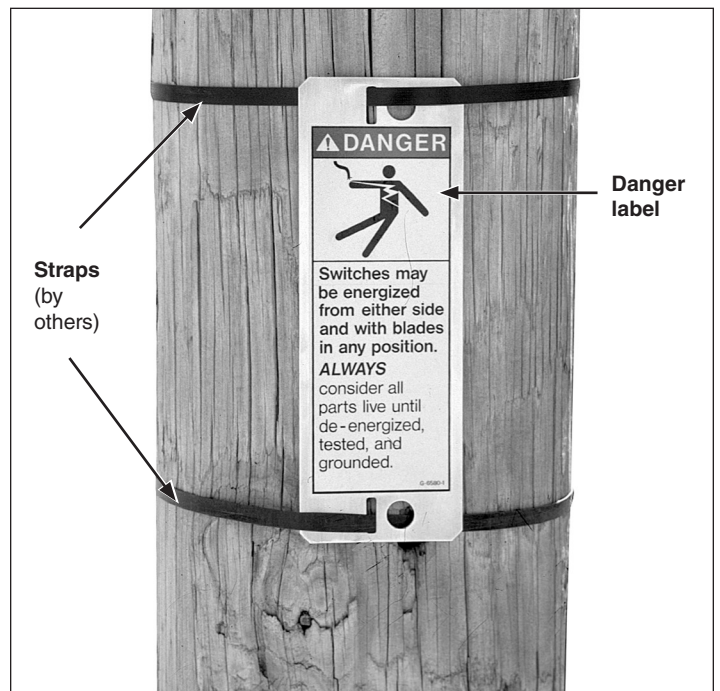
Figure 22. Attach the danger label to the pole or structure.
