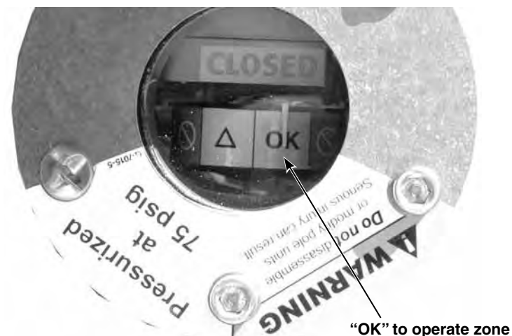
Figure 94. Check that the gas-pressure gauge on each pole-unit is in the “OK” to operate zone.
