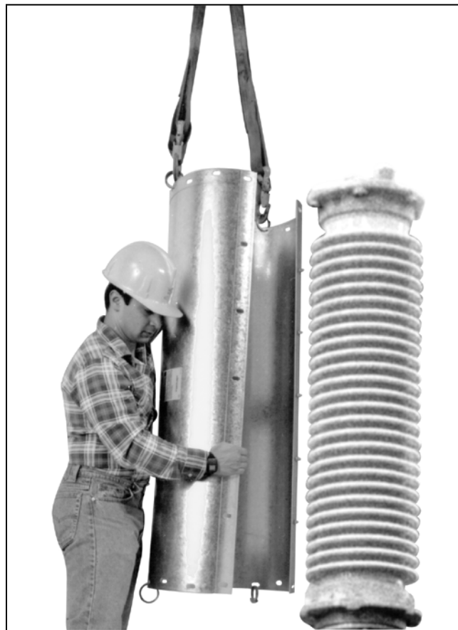
Figure 2. Raising a spare interrupter container into position on an interrupter being replaced. Model 2030 circuit-switcher illustrated; Model 2020 is similar.
