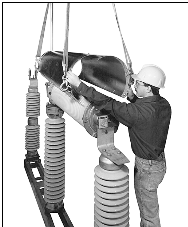
Figure 12. Raising a spare interrupter container into position on an interrupter being replaced. Model 2010 circuit-switcher illustrated; Model 2040 is similar.
