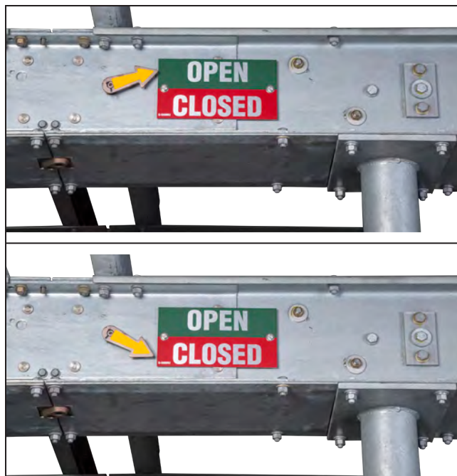
Figure 31. Switch-position indicator in the OPEN position. Switch-position indicator in the CLOSED position.
