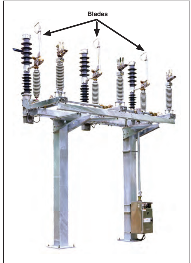
Figure 81. Disconnect blades in Open position.
