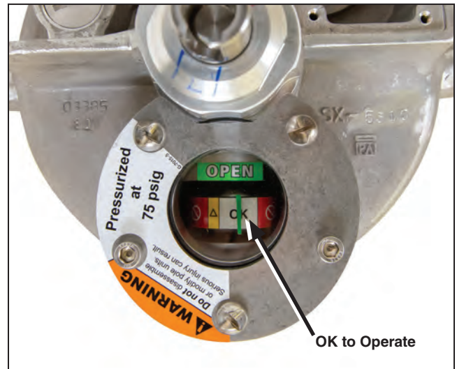
Figure 82. Make sure the indicator reads "OPEN." Make sure the gas-pressure gauge on each interrupter is in the OK to Operate zone.
