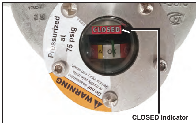
Figure 72. The interrupter is Closed and Charged. The indicator shows “CLOSED.”
