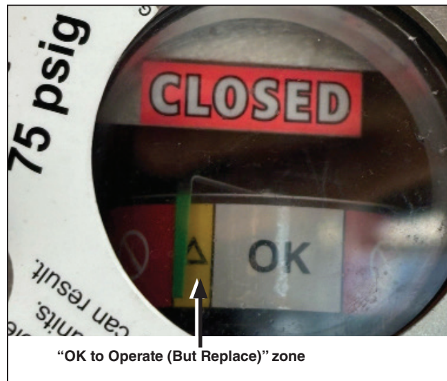
Figure 6. Gauge needle in the yellow OK to Operate (But Replace) zone.
