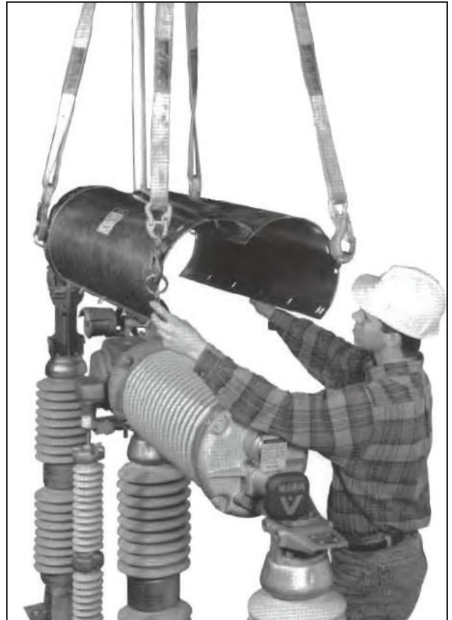
Figure 4. Raising the spare interrupter container into position. Vertical-break style circuit-switcher shown; the center-break style is similar.
