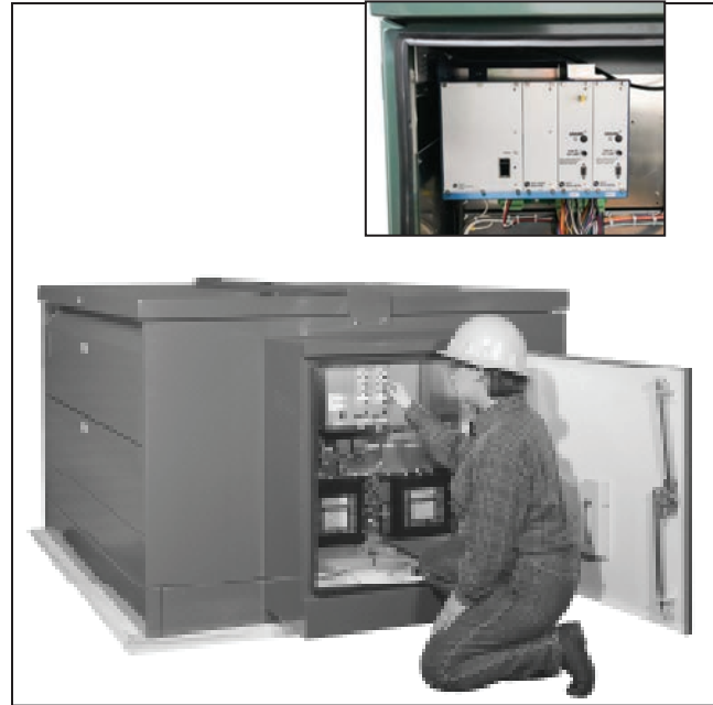
Figure 40. The location of the motor operator controls.
