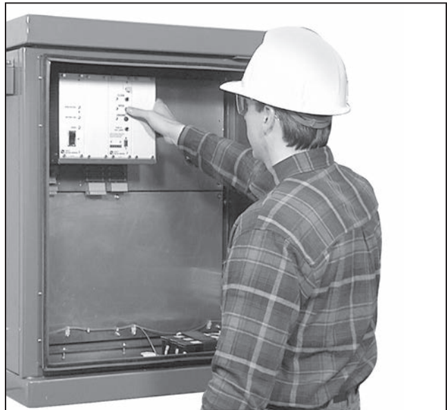
Figure 106. A vault-style low-voltage enclosure shown with provisions for a remote terminal unit and communications.
