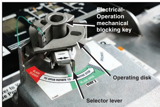
Figure 100. Close position indication on motor operator.
