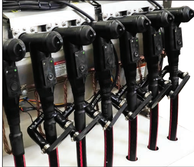
Figure 114. Wiring is already attached to the current sensors.
