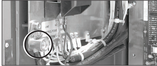
Figure 94. Copper lug and fuse block.
