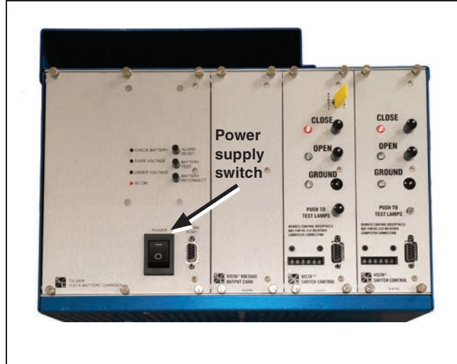
Figure 131. There are two Vista rack options, depending on the control configuration. One rack has OPEN, CLOSE, and GROUND indicators and controls; the other has only a GROUND indicator and control.
