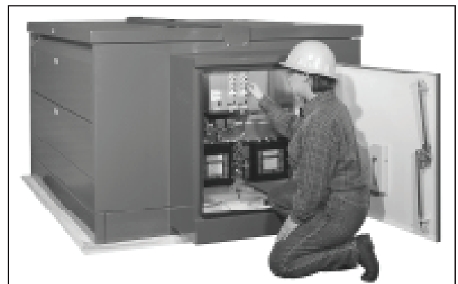
Figure 104. The location of the motor operator controls.
