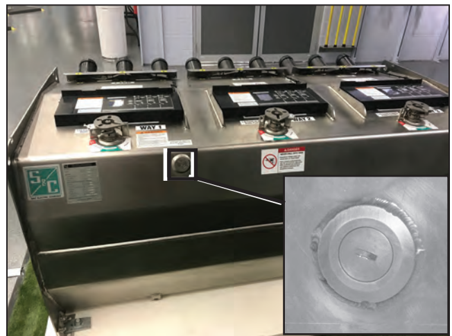
Figure 8. Location of fill port on Vista Green switchgear tank. Slotted accessible fill port shown.
