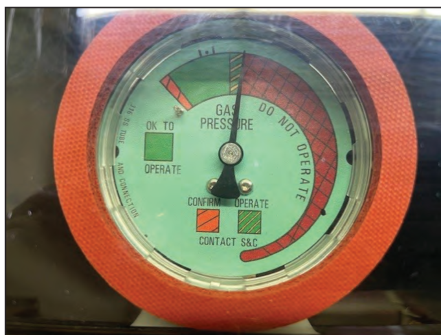
Figure 2. Vista Green Switchgear gas gauge in Green/Yellow zone.
