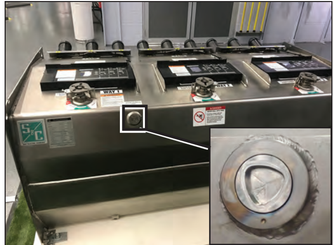
Figure 7. Location of fill port on Vista Green switchgear tank. Inaccessible fill port shown.
