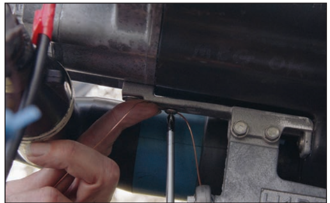
Figure 23. The bushing well interrupter grounding point.
