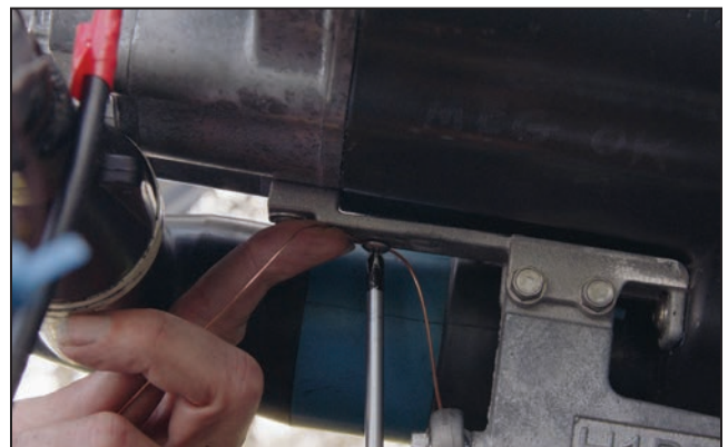
Figure 7. The bushing well interrupter grounding point.
