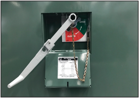
Figure 3. The access cover open and the folding switch operating handle installed.
