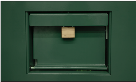
Figure 2. Switch access cover padlock.
