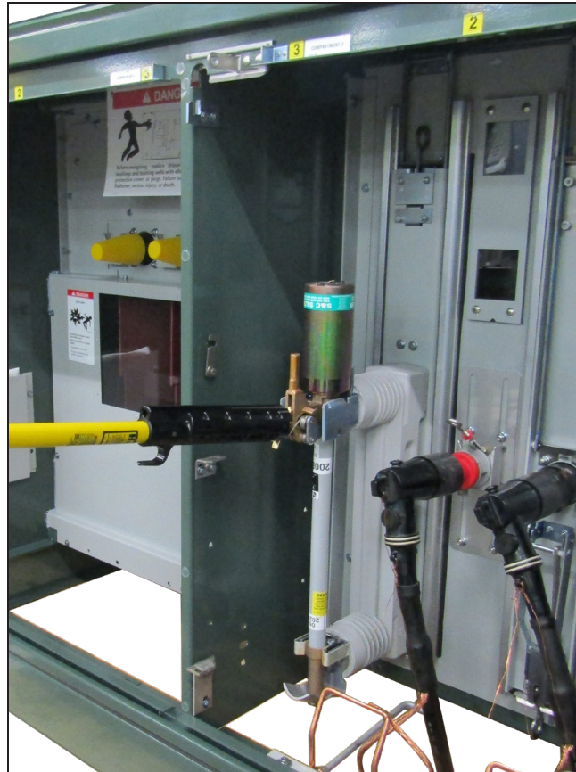
Figure 23. A shotgun stick secured to a fuse pull-ring in preparation for unlatching the fuse.
