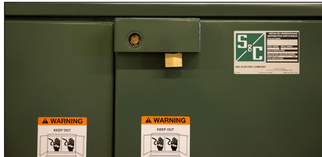
Figure 8. The enclosure doors padlocked.
