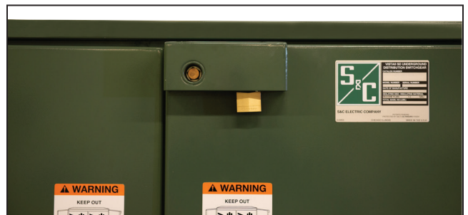
Figure 8. The enclosure doors padlocked.
