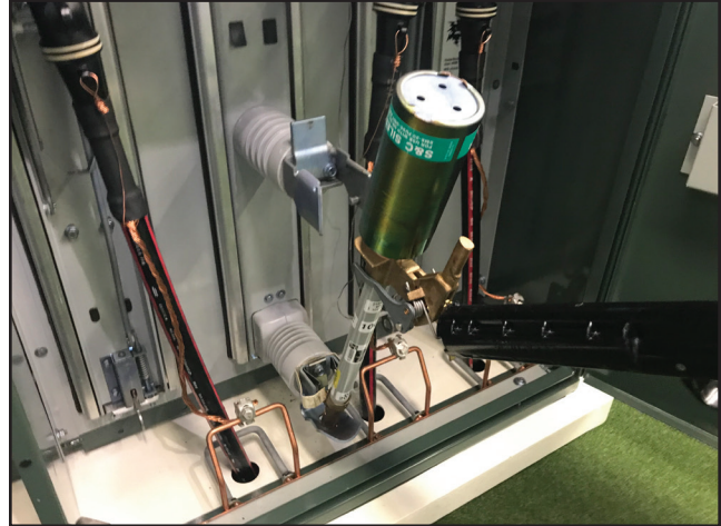
Figure 18. A fuse lowered into the cradle in preparation for latching to a TransFuser Mounting.
