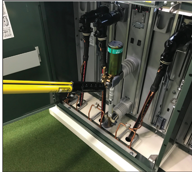
Figure 21. A shotgun stick secured to a fuse pull-ring in preparation for unlatching the fuse.
