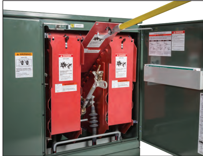
Figure 28. Inserting dual-purpose front barrier into the Slide In position using a Grapppler tool.
