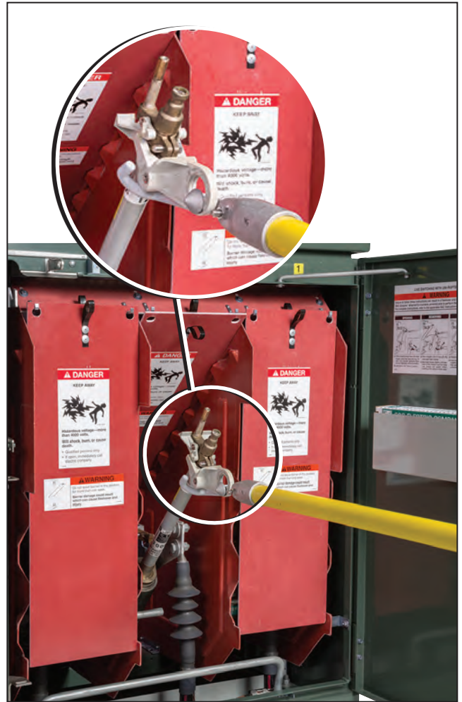
Figure 29. A Grappler tool positioned for fuse removal.
