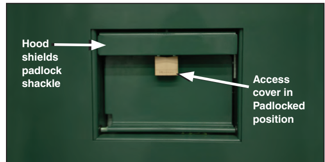
Figure 11. The access cover padlock.
