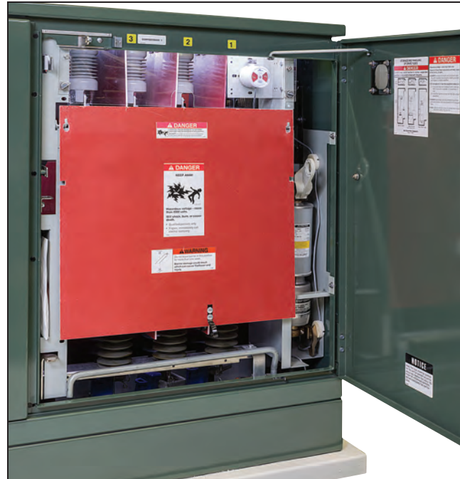
Figure 15. Dual-purpose front barrier for switch in its normal, suspended position.
