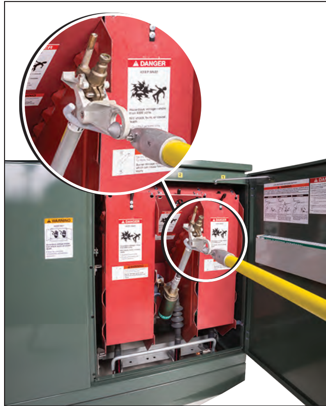
Figure 22. Installing a fuse using a Grappler Handling Tool. The inset image shows a close-up of a Grappler tool in position to install the fuse.
