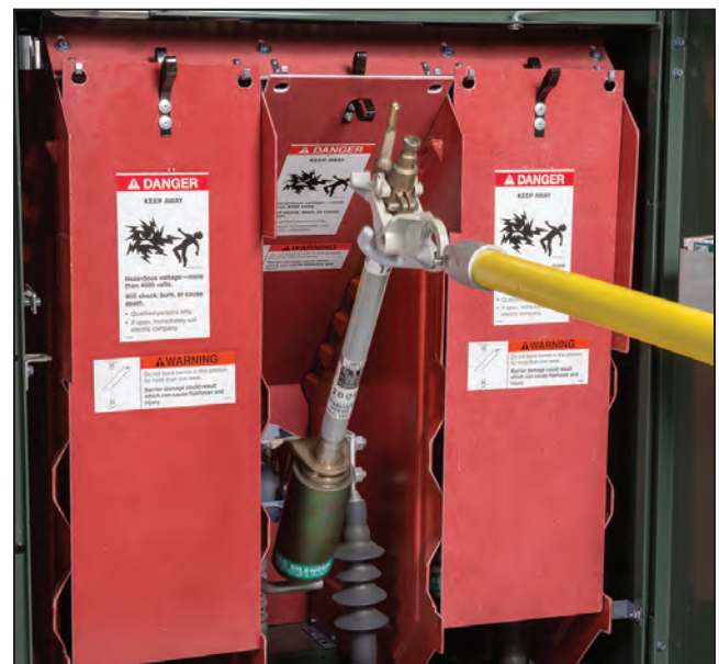
Figure 30. Removing a fuse from its hinge with a forward and upward lifting motion.
