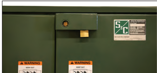
Figure 10. The enclosure doors padlocked.
