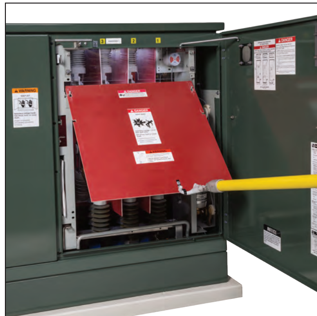
Figure 16. A Grappler Handling Tool being used to lift the barrier. Note the door holder is in place and the adjacent door is latched closed to reduce exposure to high voltage.
