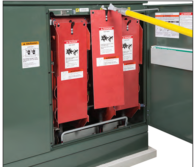
Figure 20. Removing or replacing the dual-purpose front barrier with the Grappler tool.
