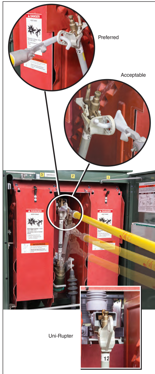
Figure 25. Closing the fuse with a swift, unhesitating stroke. The top left inset shows a close-up of a Grappler tool in the preferred position to close the fuse. The top right inset shows a close-up of a Grappler tool in an acceptable position to close the fuse. The bottom inset shows a close-up of a Uni-Rupter Interrupter with the fuse fully closed.
