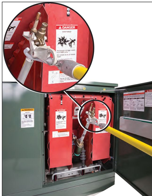
Figure 22. Installing the fuse using the Grappler tool. The inset image shows a close-up of the Grappler tool in position to install the fuse.
