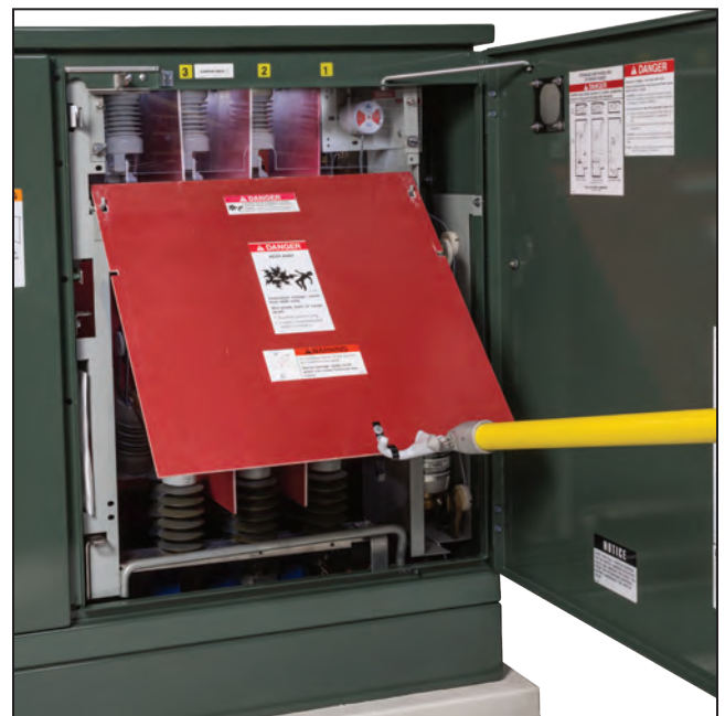
Figure 16. The Grappler tool being used to lift the barrier. Note: The door holder is in place and the adjacent door is secured closed to reduce exposure to high voltage.
