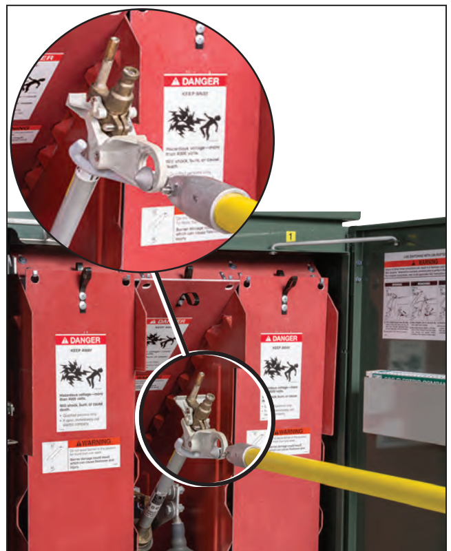
Figure 29. The Grappler tool positioned for fuse removal.
