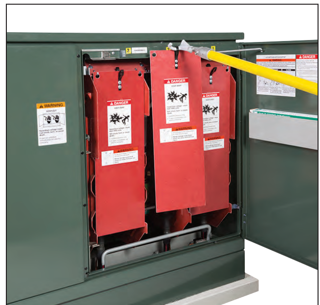
Figure 20. Removing or replacing the dual-purpose front barrier with the Grappler tool.
