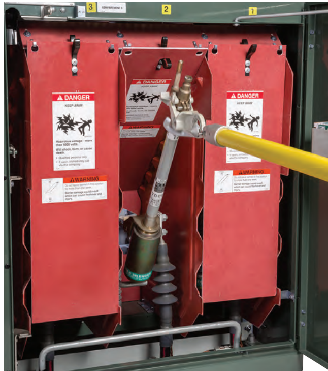
Figure 30. Removing a fuse from its hinge with a forward and upward lifting motion.
