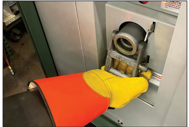
Figure 12. Decoupler handle being moved upward to decouple the switch from the associated switch operator.
