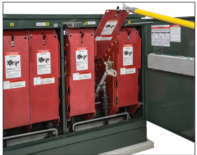
Figure 24. Removing the dual-purpose front barrier from the Slide In position using a Grappler tool.
