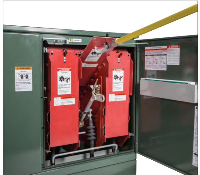
Figure 28. Inserting the dual-purpose front barrier into the Slide In position with the Grappler tool.
