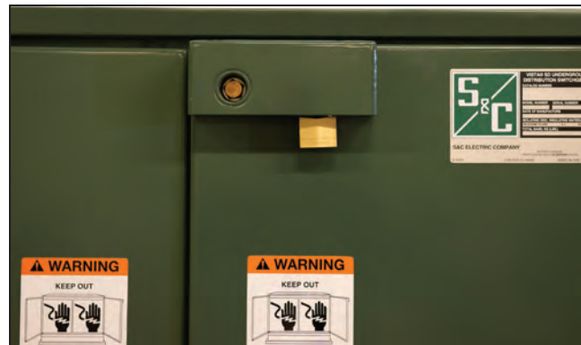
Figure 11. The enclosure doors padlocked.
