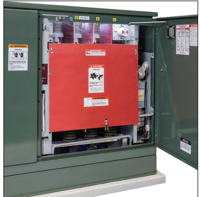
Figure 15. The dual-purpose front barrier for the switch in its normal, suspended position.
