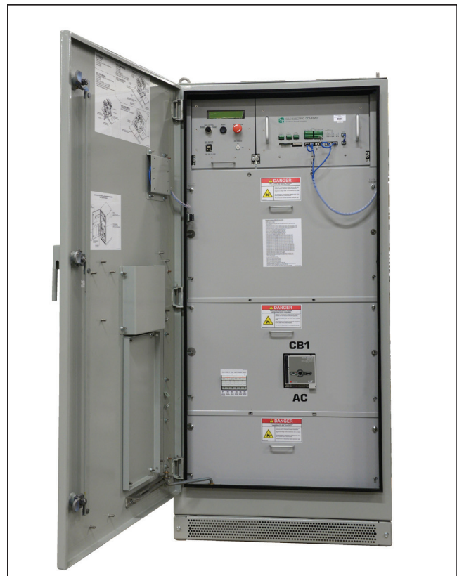
Figure 2. Internal view of the power conversion system.
