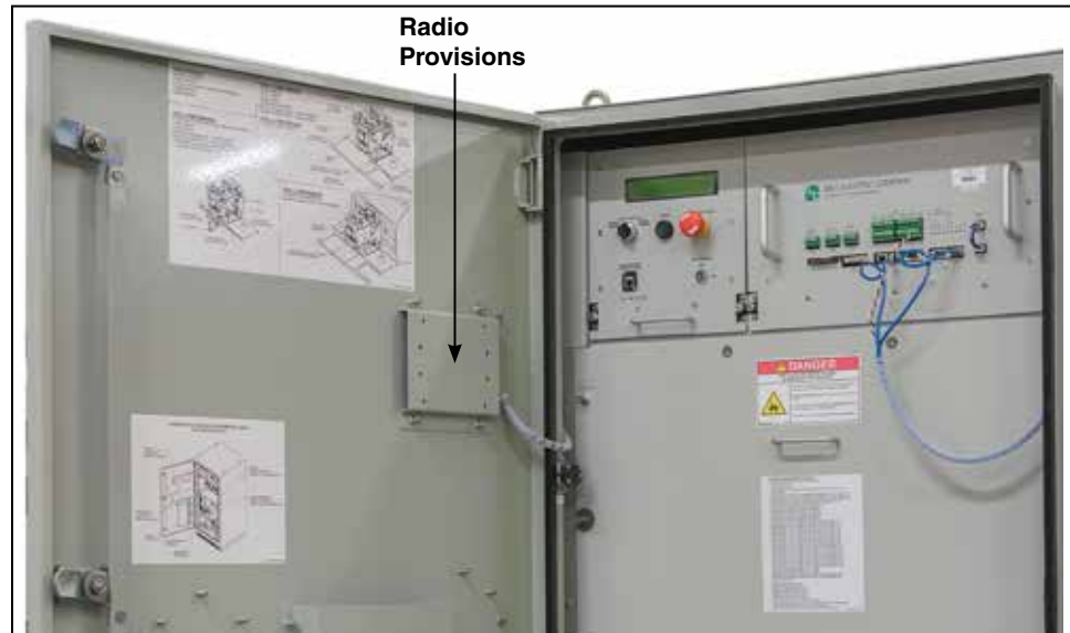
Figure 16. Provisions for radio communication.
