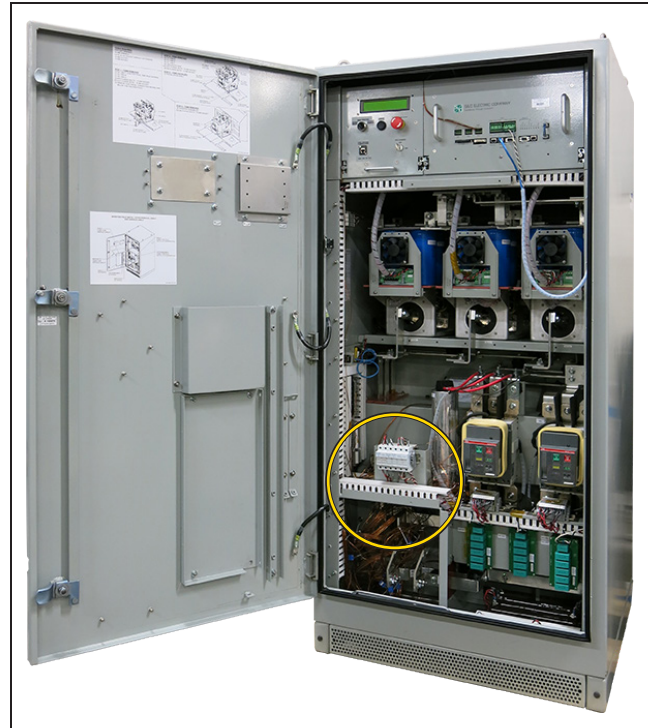
Figure 6. Location of the cable termination area.
