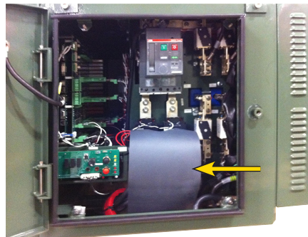
Figure 1. Shield protection from wiring (front of unit).
