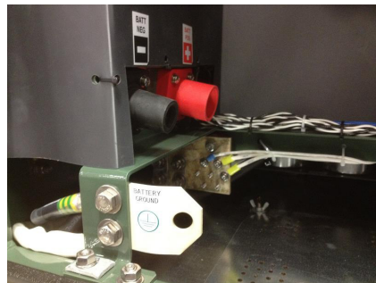
Figure 3. Visible battery non-load-break disconnect terminals.
