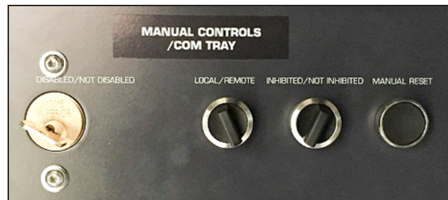
Figure 5. Control panel on the master control rack.
