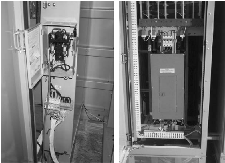
Figure 14. 110-Vac, 30-A safety switch configuration (left), 208-Vac panel board for larger, outdoor applications (right).
