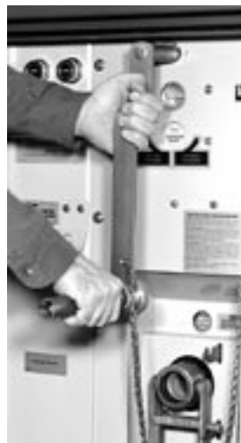
Figure 19. Dual purpose manual handle inserted in the groove of shaft for emergency manual switching.
