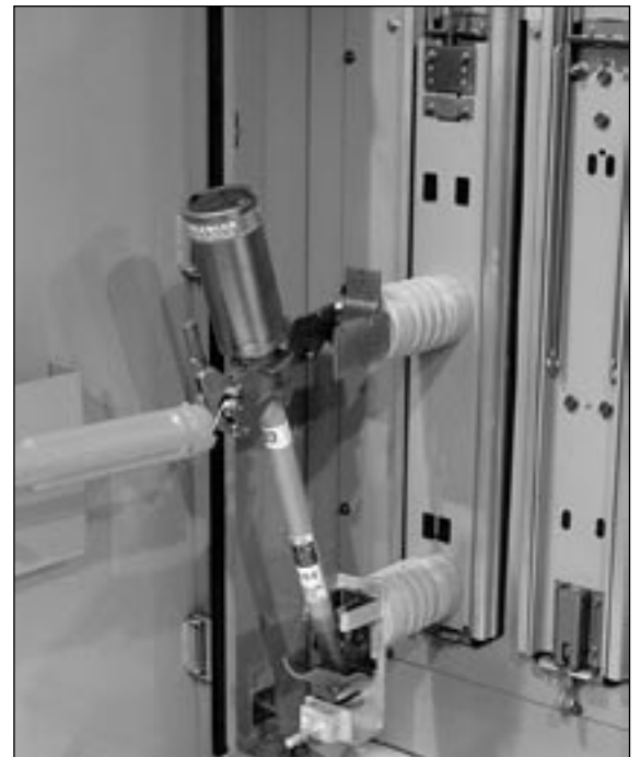
Figure 8. Fuse lowered into the cradle in preparation for latching to fuse access panel.
