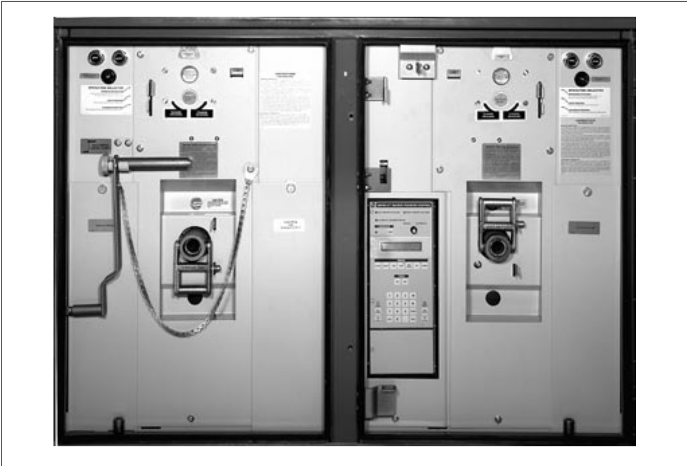
Figure 15. Low-voltage control compartment.
