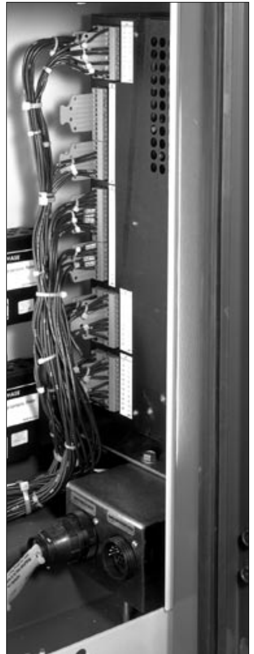
Figure 17. Access panel removed showing input plug, input receptacle, and shunting receptacle of S&C Micro-AT Source-Transfer Control.
