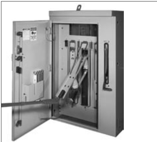
Figure 4. To replace the fuses, pull the ring at the bottom of the TransFuser panel.
