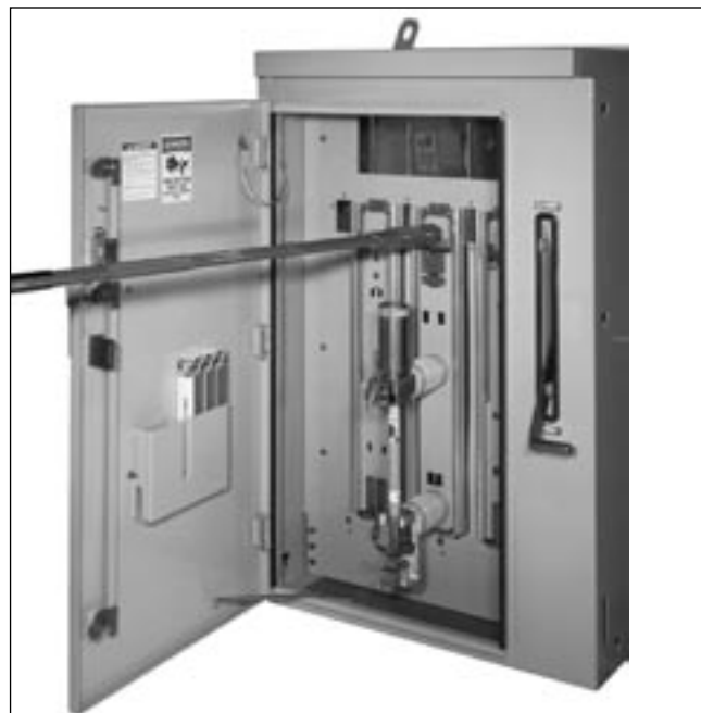
Figure 6. The fuse, now in full view and completely separate from the bus, can be easily removed from the mounting.
