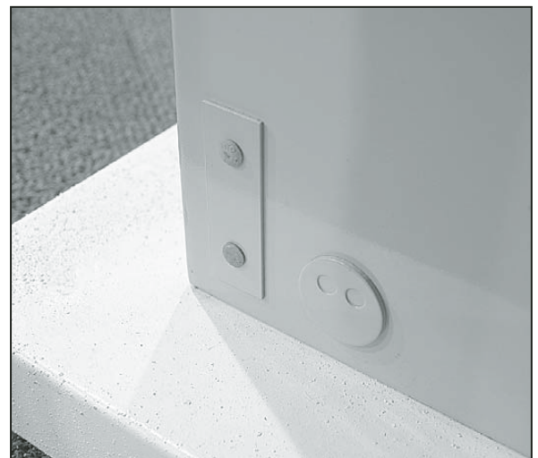
Figure 27. Exterior view of ground bus plate on existing end module.
