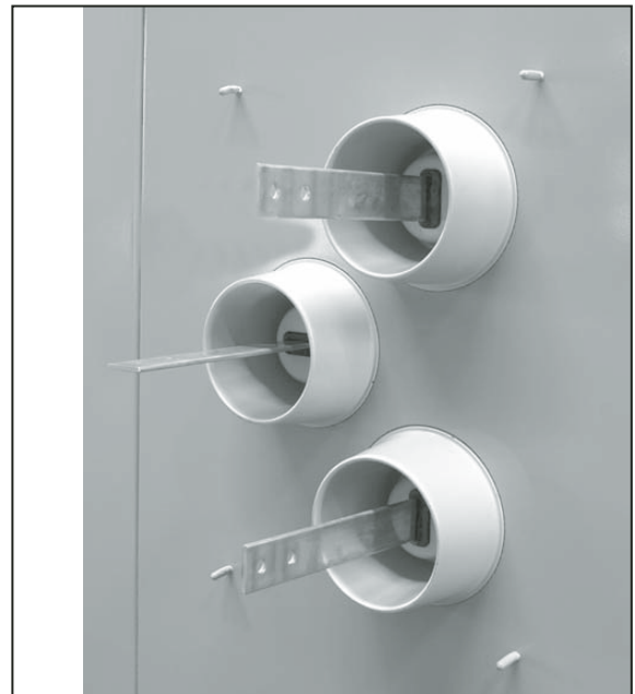
Figure 12. Grommets on the through-bushings.
