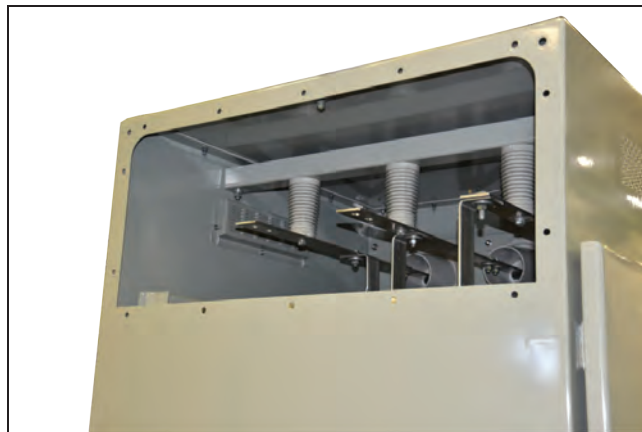
Figure 8. Bolt and nut location at the edges of the through-bus openings.
