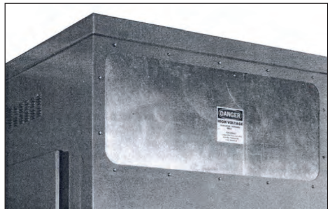
Figure 18. The end plate removed to accept a new unit leaving the inner protective barrier exposed.
