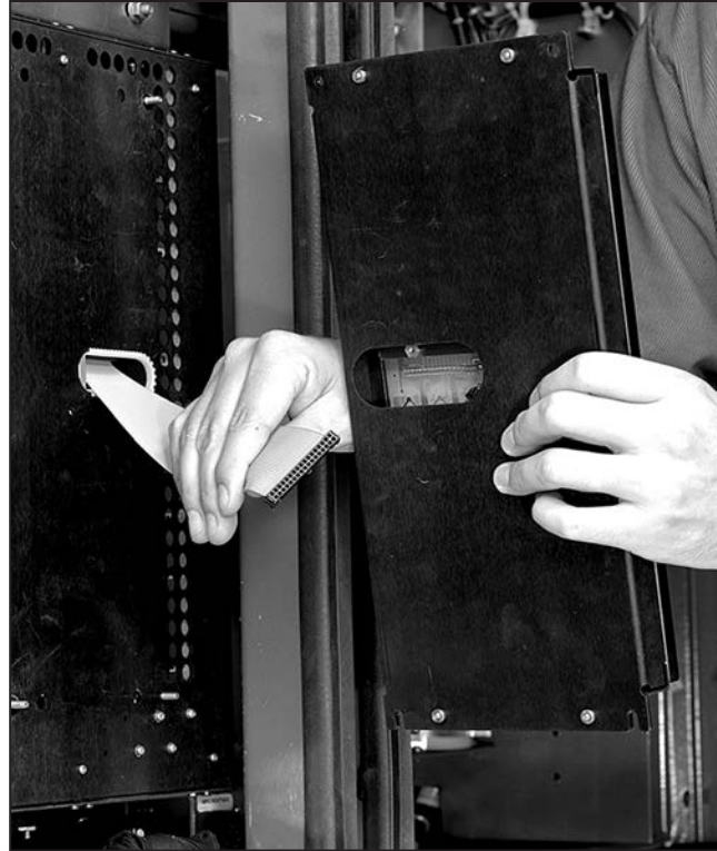
Figure 6. Disconnecting the ribbon connector plug from the receptacle on the front panel assembly in pad-mounted gear originally furnished with a Type AT-12 Source-Transfer Control.
