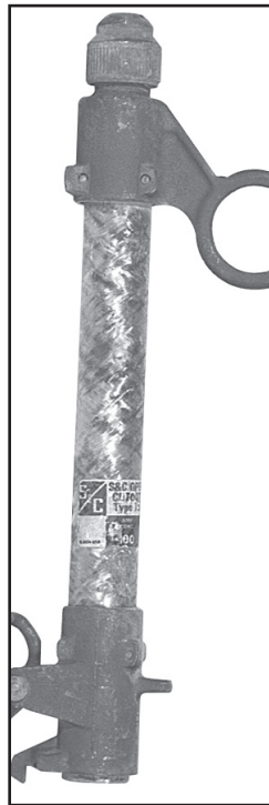
Figure 1(b). Acceptable: Paint is completely faded.
