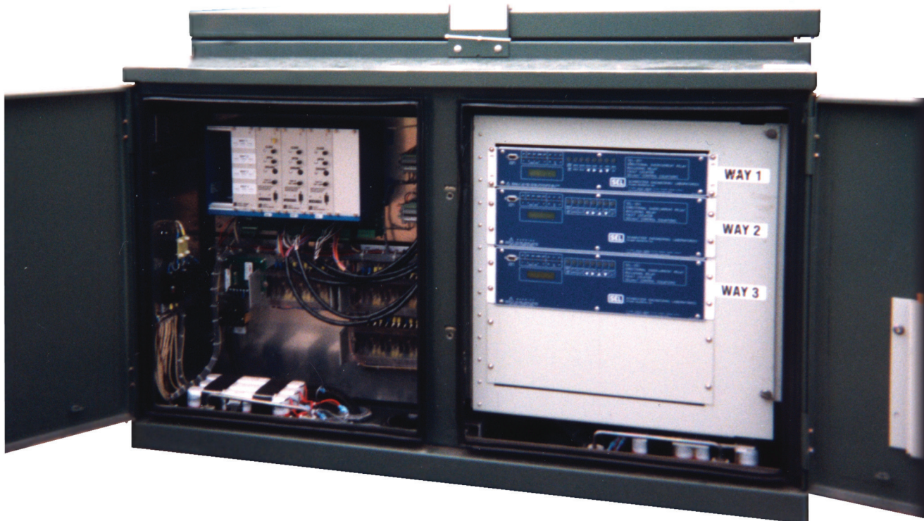
Figure 2. SEL-351 Relays housed in the low-voltage compartment of Vista Underground Distribution System.
