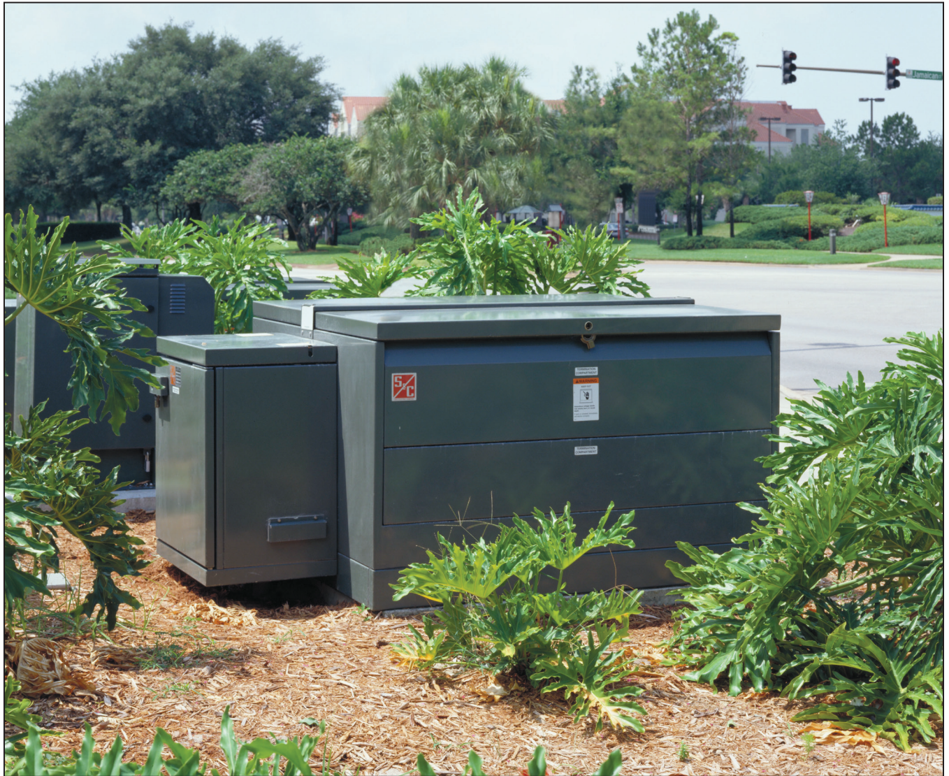
Figure 1. Remote Supervisory Vista Underground Switchgear.
