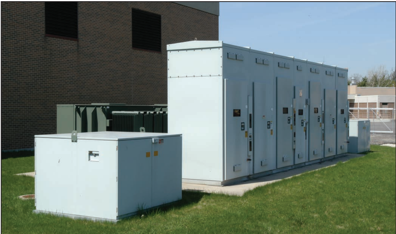
Figure 4. Metal-Enclosed Switchgear providing switching and protection to a wastewater treatment facility.
