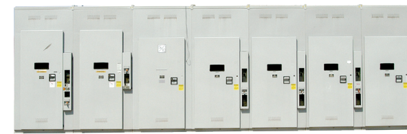
► 20a Custom Metal-Enclosed Switchgear with Micro AT® Source-Transfer Control
