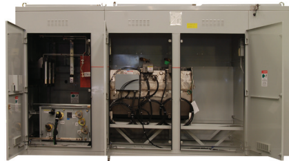
Front and rear access, primary metering, cables from below
