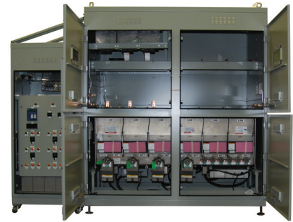
Front access only, cables from above
