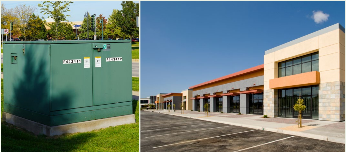
FIGURE 6. This large suburban shopping mall is served by seven units of pad-mounted gear in two looped-primary circuits. Two lineups of metal-enclosed switchgear are applied at primary-selective service-entrance switching centers to switch the ends of the loops.
