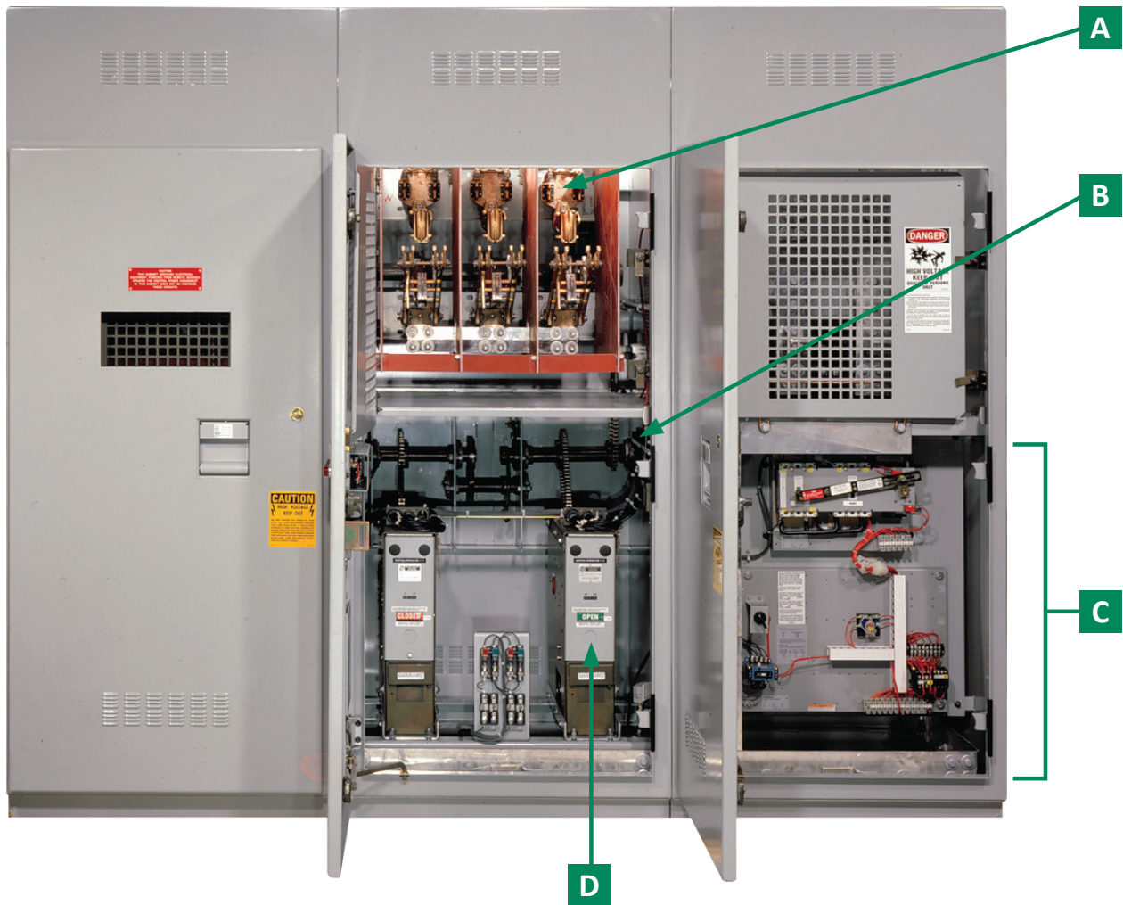
FIGURE 8. Three-bay, custom, power-operated, indoor, switchgear assembly with remotely operated interrupter switches in left-hand and center bays and a mechanical cam interlock in the center bay for sequencing of switch operations. Bay at right is a bus-tap entrance with low-voltage components at the bottom.
