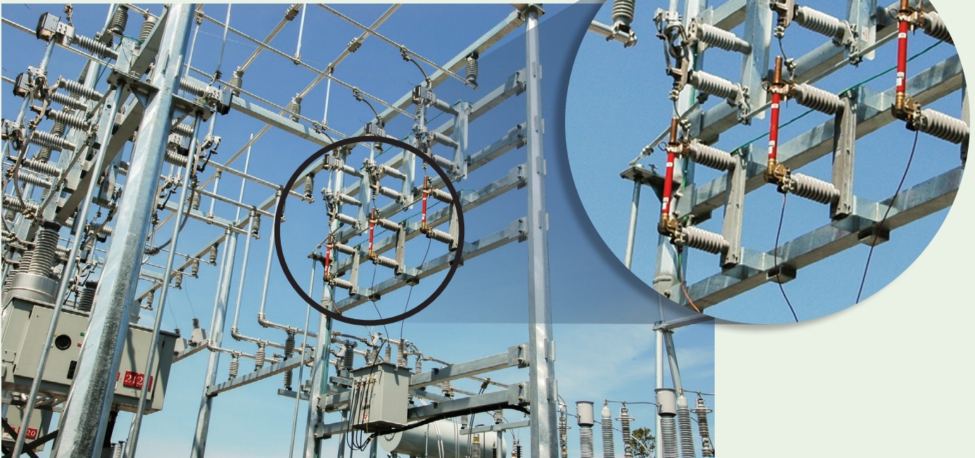
FIGURE 2. Transformer protection using three vertical, 180° opening-style SMD Power Fuses.
