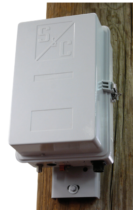
Figure 5. SpeedNet Utility-Pole-Mounted Repeater Radio.
