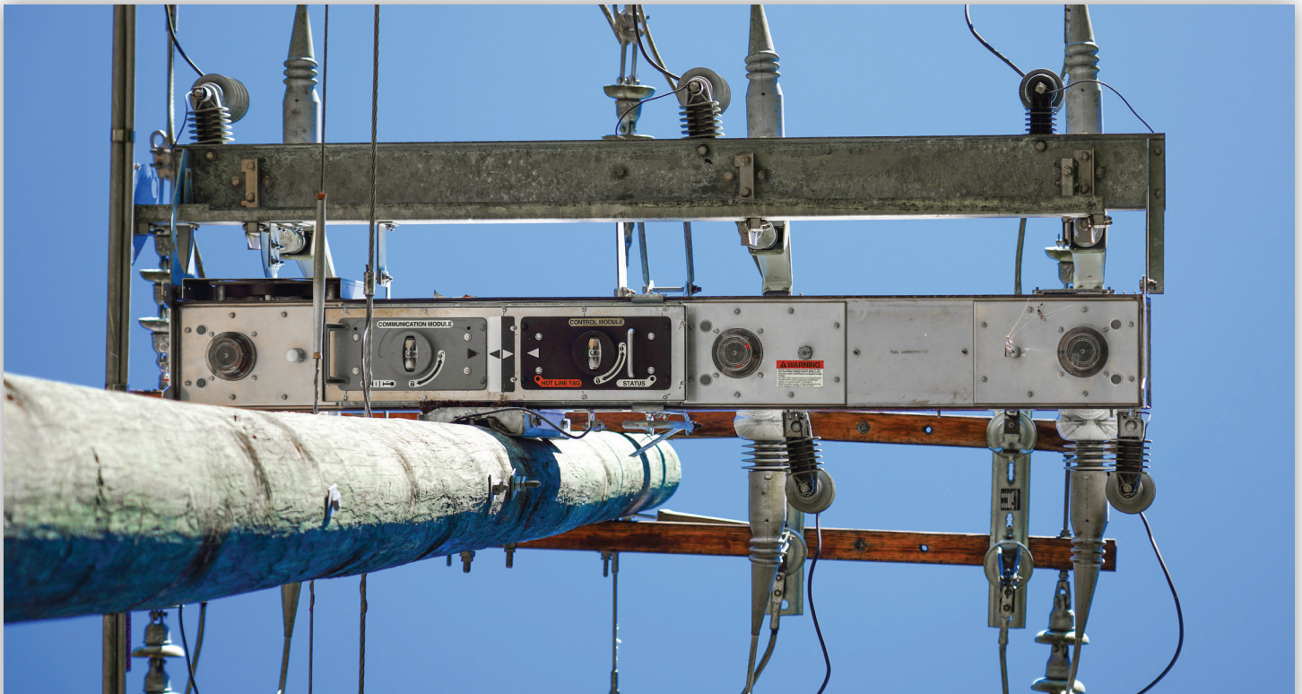
FIGURE 1. IntelliRupter fault interrupters helped Ameren Missouri increase its feeder segmentation.
