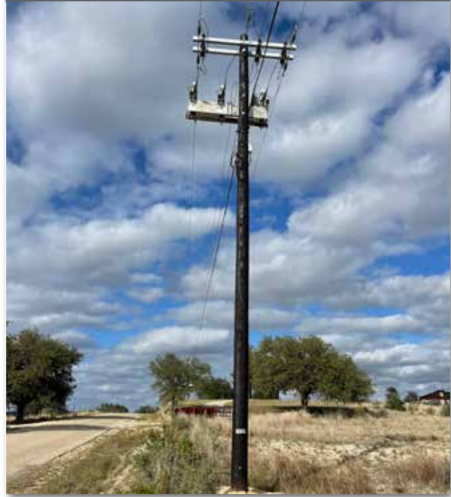
An IntelliRupter fault interrupter installed on BEC's system.
