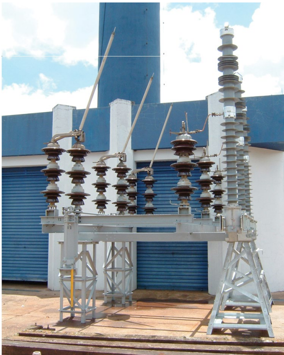
FIGURE 1. A Trans-Rupter II Transformer Protector with a disconnect on a mobile base.
