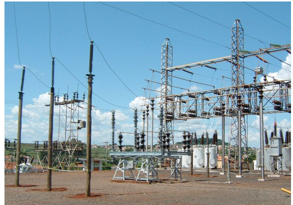
FIGURE 2. A Trans-Rupter II Transformer Protector with a mobile unit as a protective bypass for a circuit breaker during maintenance.
