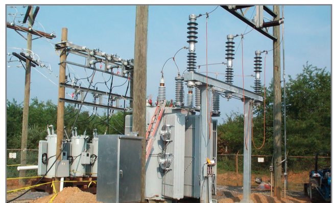
The Trans-Rupter II Transformer Protector Model EX during installation.
